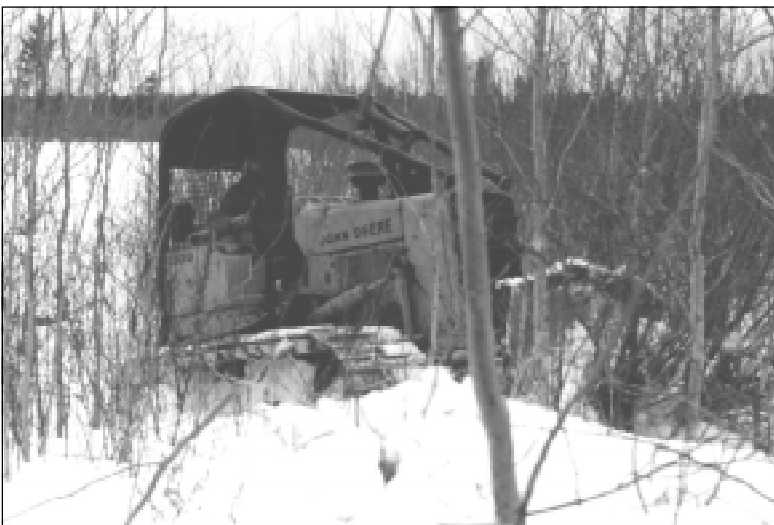
In the mechanical strip thinning process, an eight-foot-wide strip of aspen is bulldozed to encourage the remaining trees to grow faster.
